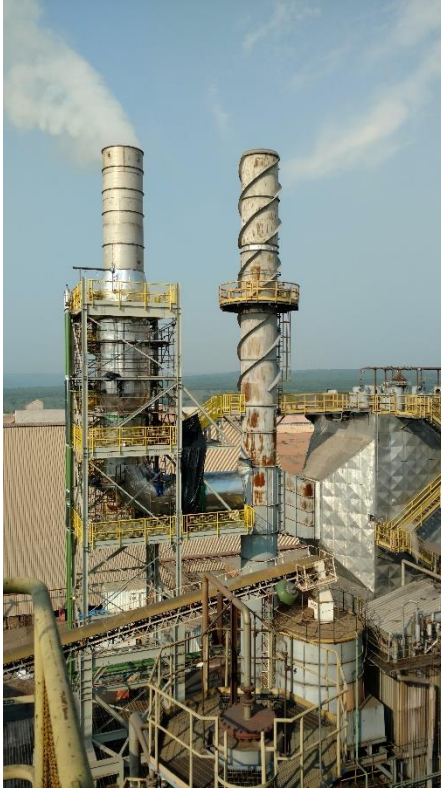
Wood Fired Boiler Exhaust Heat Recovery
