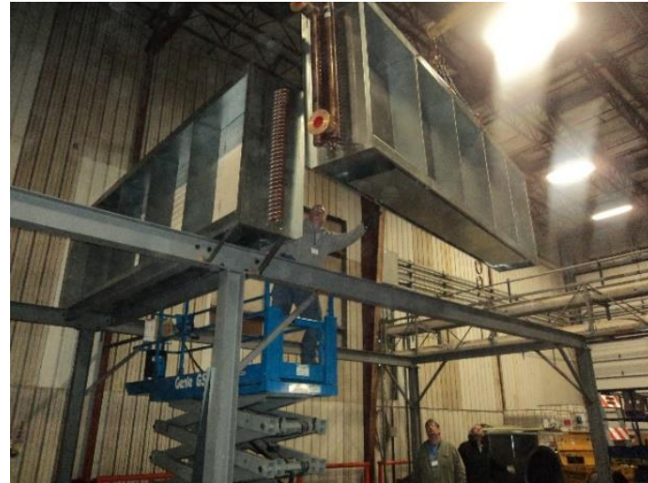
Scrubber Exhaust Heat for Makeup Air Preheating
