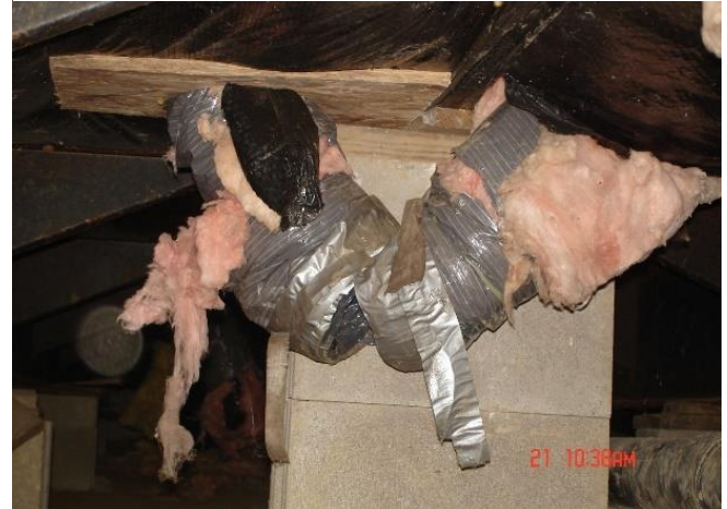
Figure 8. Example of a failed cross-over duct connection under a multi-section manufactured home.
