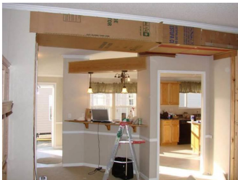
Figure 16. Interior duct chase mock up by Southern Energy Homes (Moyer, et al. 2008)
