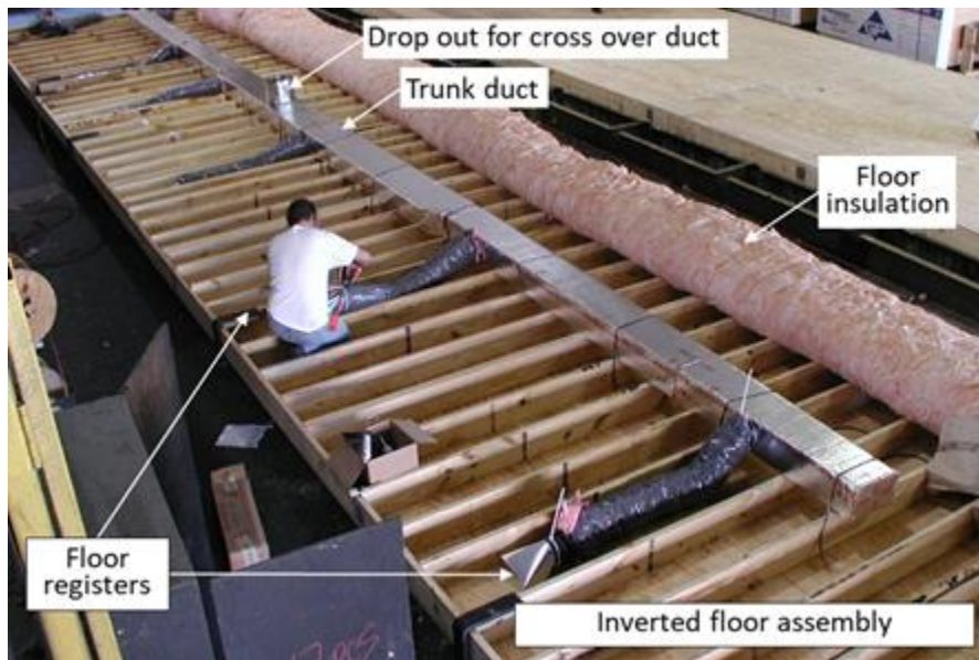
Figure 13. Duct system being installed on an inverted floor section that will be flipped over once completed
