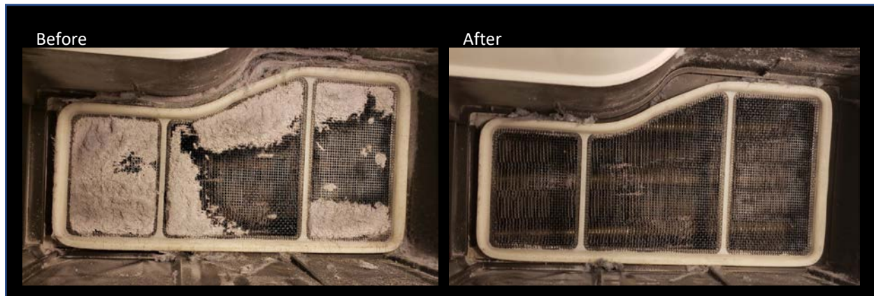
Figure 25. View of coarse screen located downstream of the secondary lint filter on the Whirlpool full-size heat pump dryer, before and after cleaning (Site 6). The heat pump evaporator coils are visible behind the screen.
