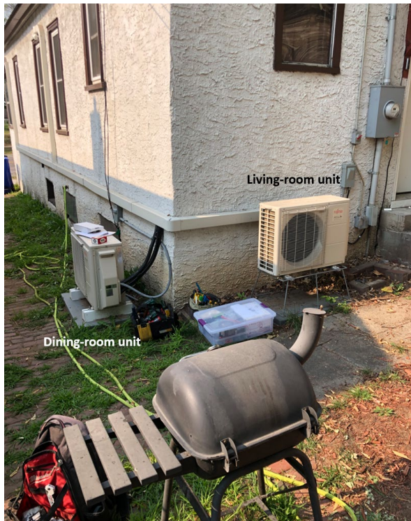
Figure 6. Exterior view of the Site 1 home showing the outdoor units for the two mini-split systems.
