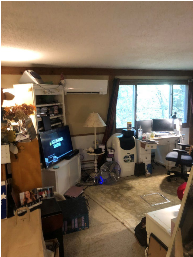
Figure 17. The indoor unit of the mini-split system at Site 3.
