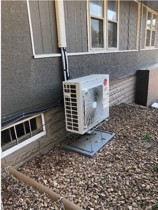
Figure 9. The outdoor unit for the Site 2 mini-split system.
