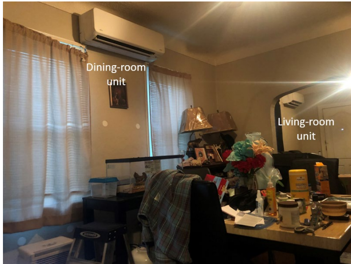
Figure 3. Interior view of two mini-split units at Site 1.
