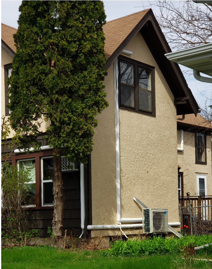
Figure 1. Example of a multi-head ductless mini-split system in Minneapolis.
