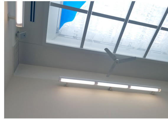
The atrium area, served by wall mounted fixtures with supplemental control modules.
