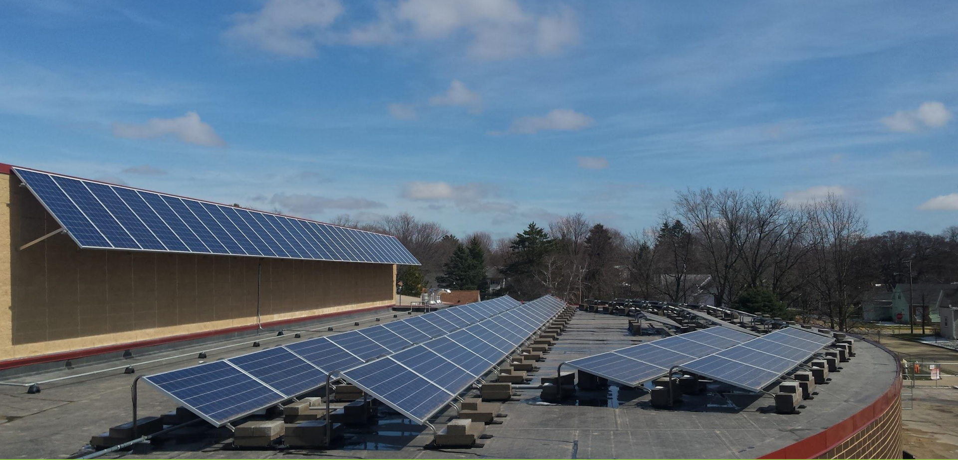
Brooklyn Elementary School Solar | 36 KW
