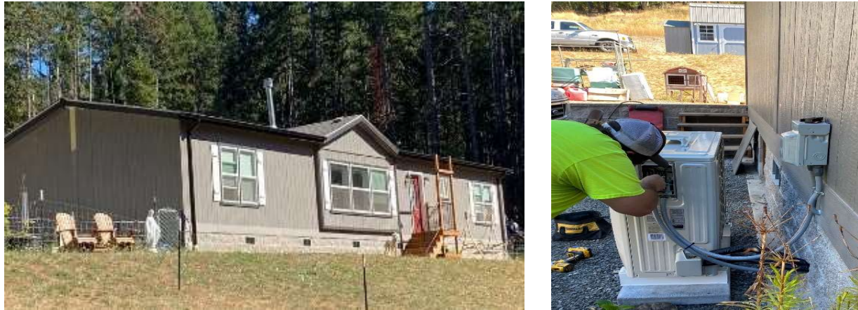
Figure 1. Picture of the manufactured home (left) and heat pump installation (right)
