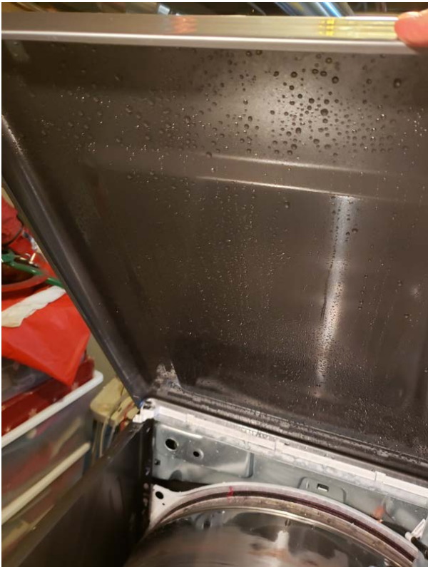
Figure 16. Moisture covering the interior of the malfunctioning heat pump dryer for Site 1.
