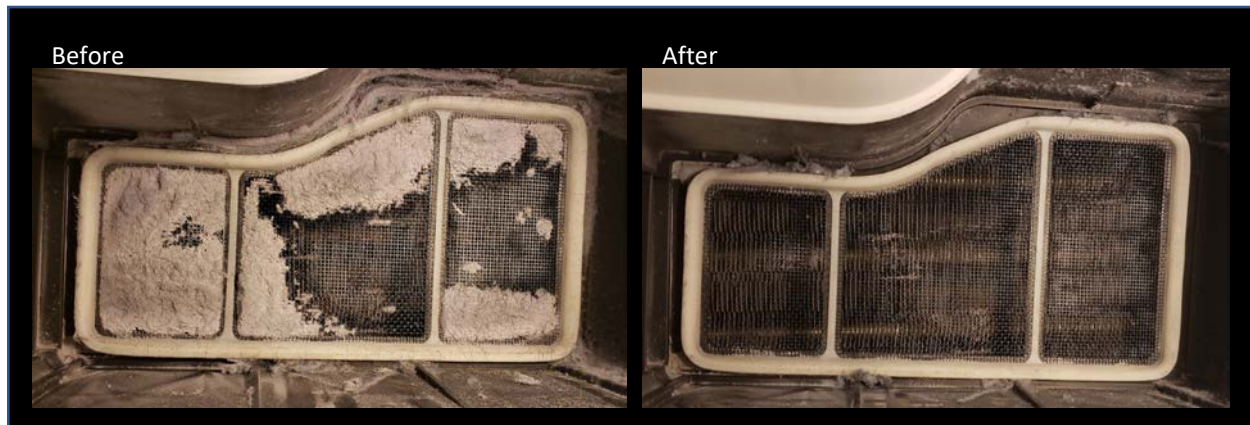
Figure 25. View of coarse screen located downstream of the secondary lint filter on the Whirlpool full-size heat pump dryer, before and after cleaning (Site 6). The heat pump evaporator coils are visible behind the screen.
